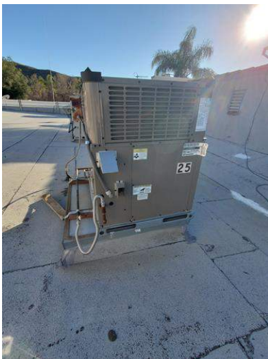
Description: September 2020, M&M, POA #25 HVAC Replacement, $7,500.
